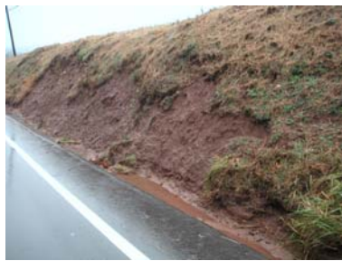
“Road creep” and sedimentation
