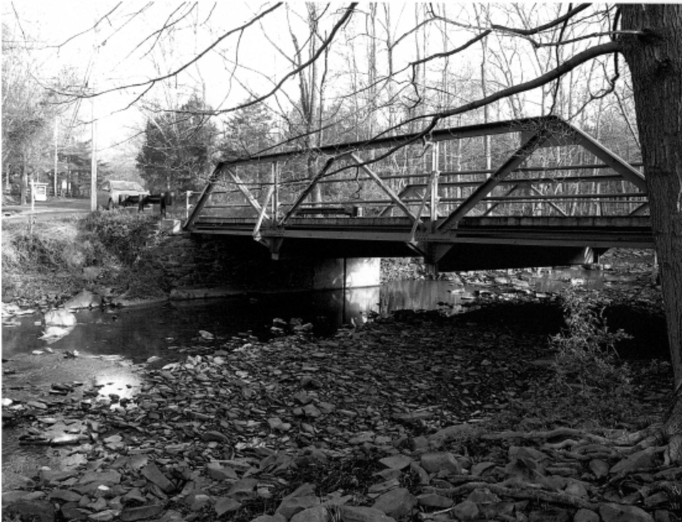
Metal Truss Bridge Example Delaware Township Historic Bridges MPDF Delaware Township, Hunterdon County, New Jersey
