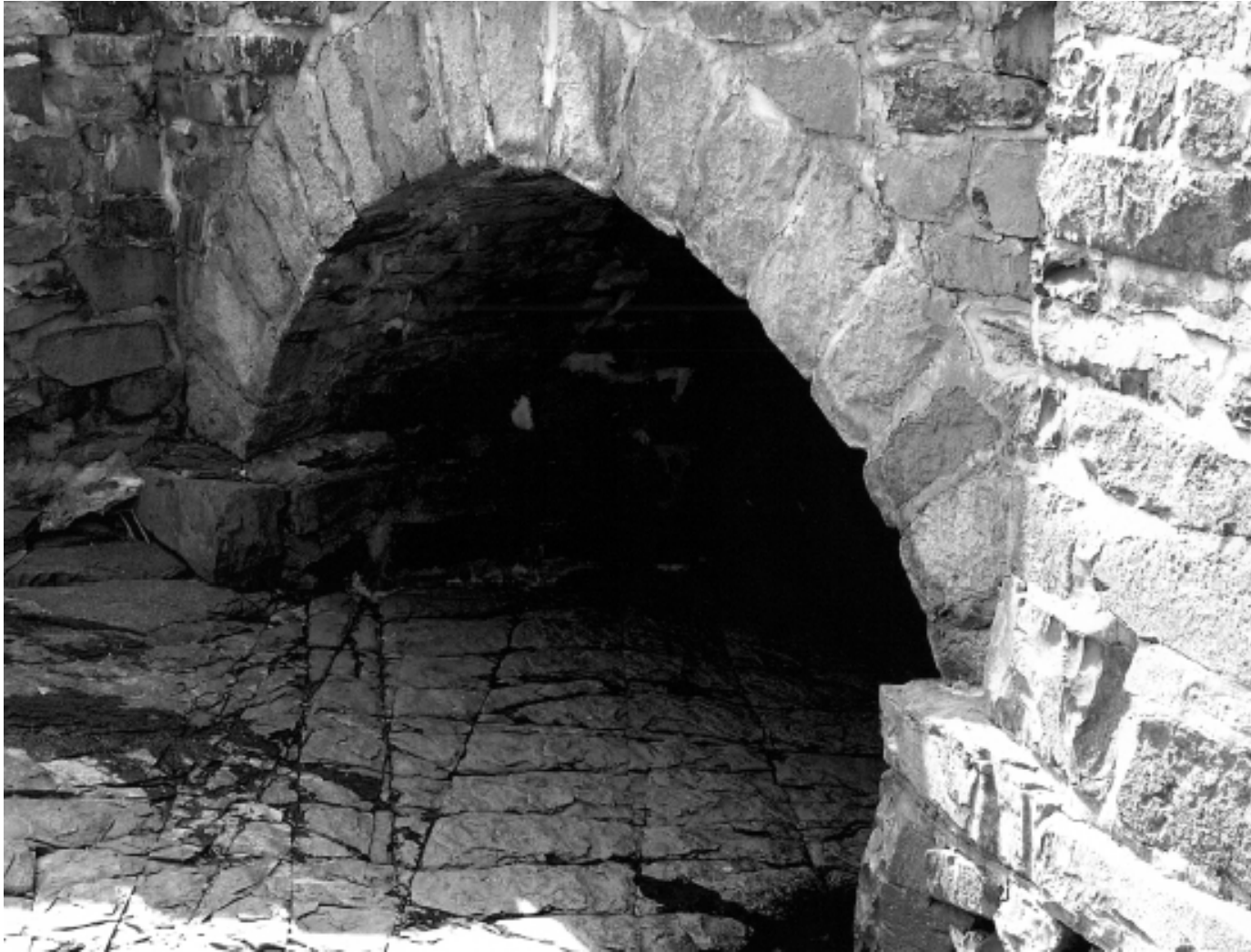
Stone Arch Bridge Example Delaware Township Historic Bridges MPDF Delaware Township, Hunterdon County, New Jersey
